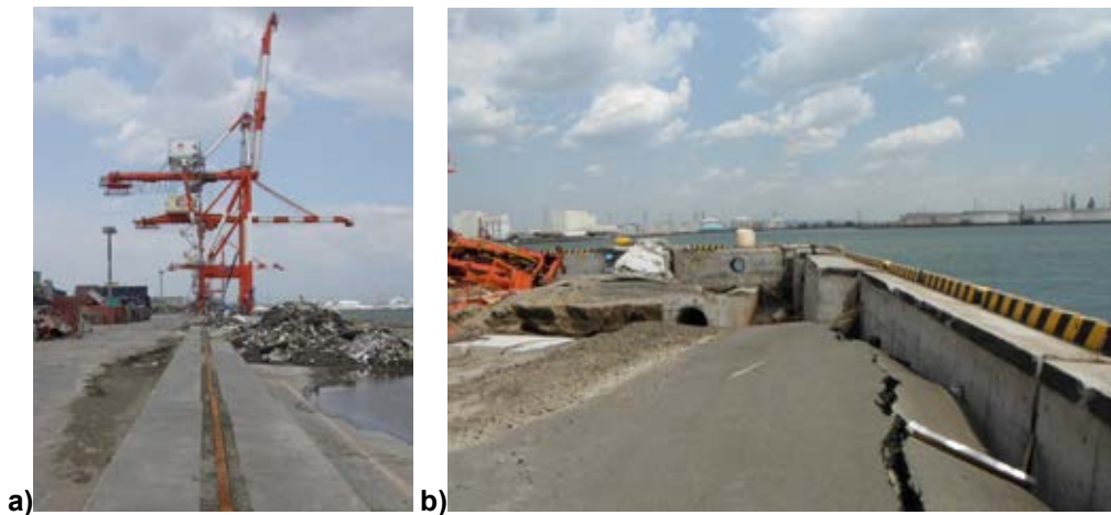
Fig. 2.3 a) Landside crane rails at the eastern side and b) Rotated wharf closure bulkhead at the east end of the Takasago wharf (Percher, 2014)
