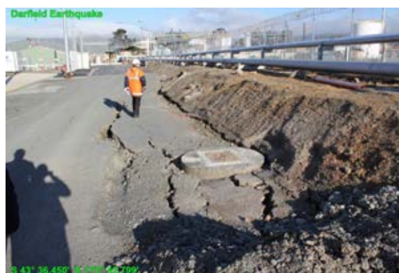
Fig. 2.4 Settlement and lateral deformation at fuel transfer facility (Cubrinovski et. al., 2010).
