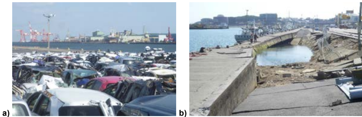
Fig. 2.1 a) Damage in Sendai port, b) Failed quay at Hitachi port (Aydan 2011)
