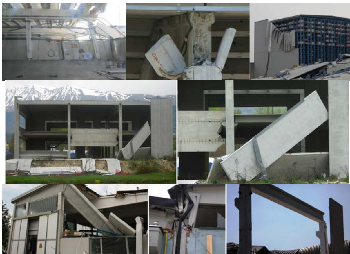
Figure 1.1: Some photos of damage to precast industrial warehouse buildings due to earthquakes including column rotation failure, cladding failure, and beam-column connection failure
